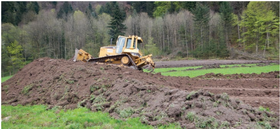
Figure 28: A negative example for soil excavation: No separation of turf, the high thickness of topsoil deposit and driving on deposit with heavy machinery (Photo: Thomas Peham).
